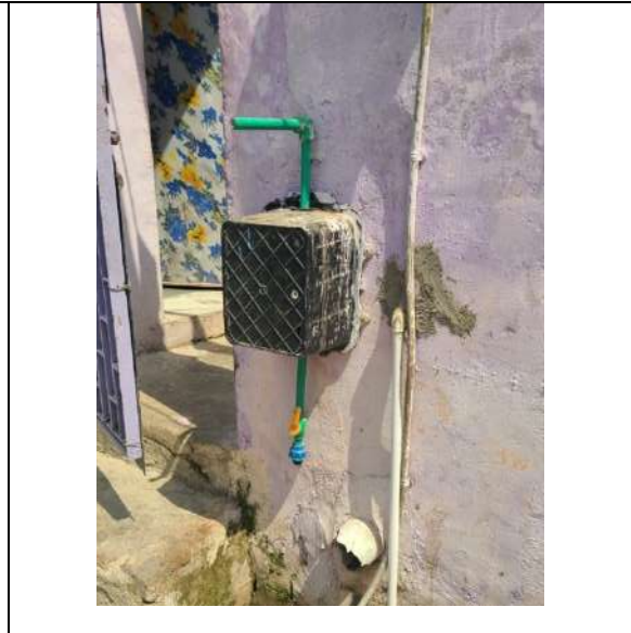
Smart Water Meters Damaged by Users
