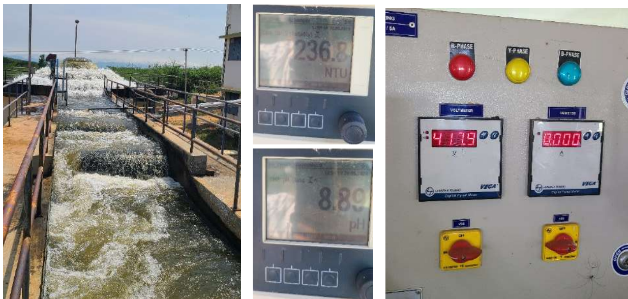
Figure 28: Cascading Aeration (left), turbidity sensor and pH sensor (middle), Flowmeter and pressure transmitter (right)
