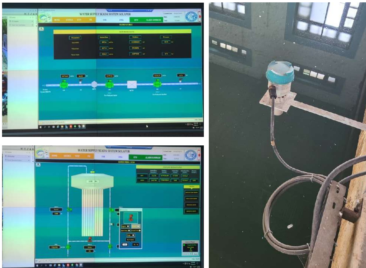
Figure 35: Monitoring of Flow and Pressure at Ujjaini Water Source
