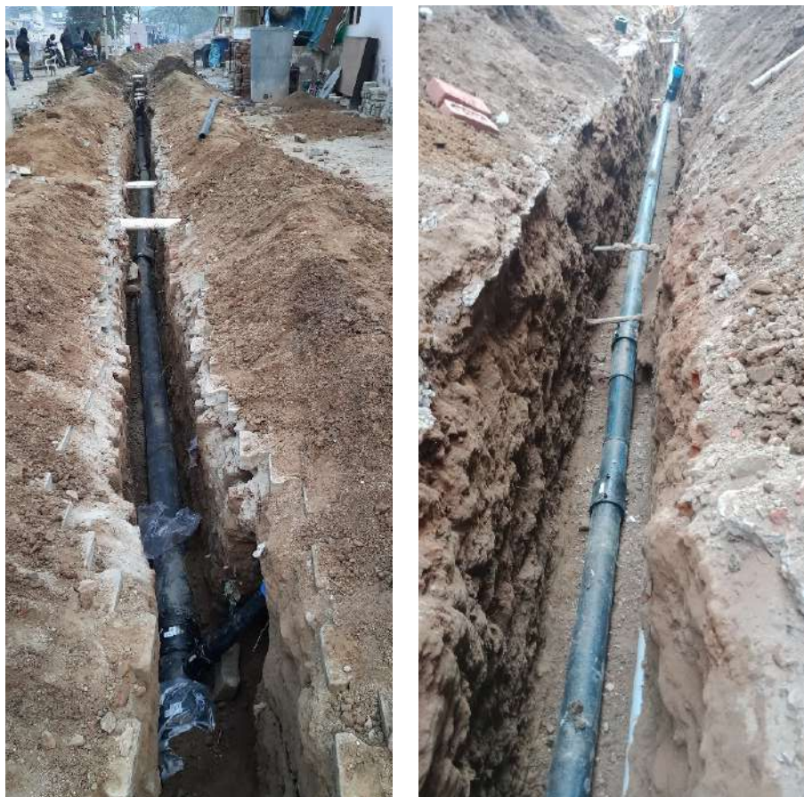
Fig 4: Vacuum Sewer Main (1.8 km)
