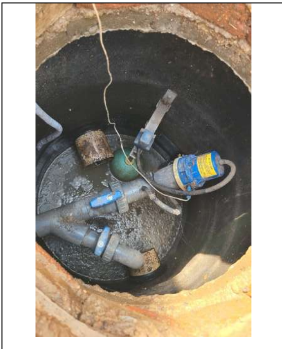
Vacuum Sewer System in Tajganj area of Agra
