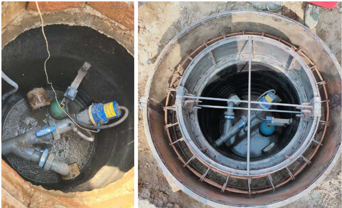
Fig 3: Smart Manholes in Tajganj, Agra
