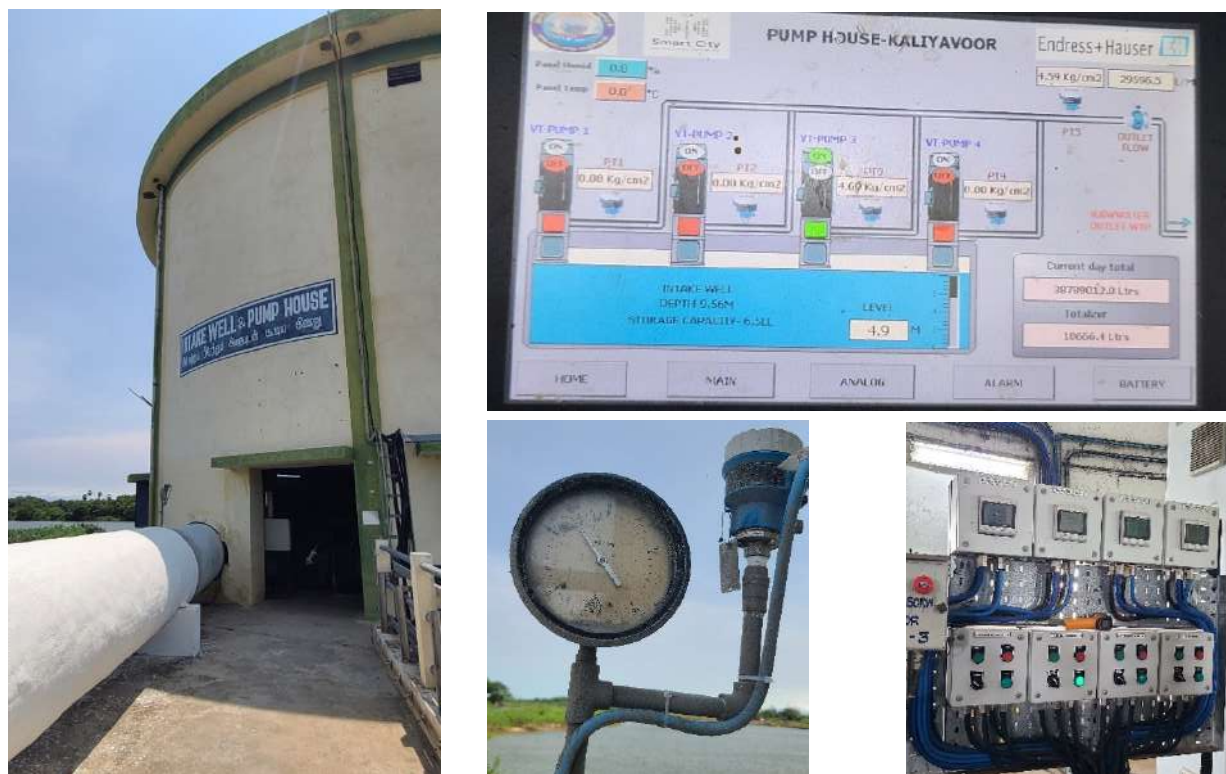
Figure 26: IoT devices and SCADA system at Kaliyavoor Treatment Plant, Source: Authors
