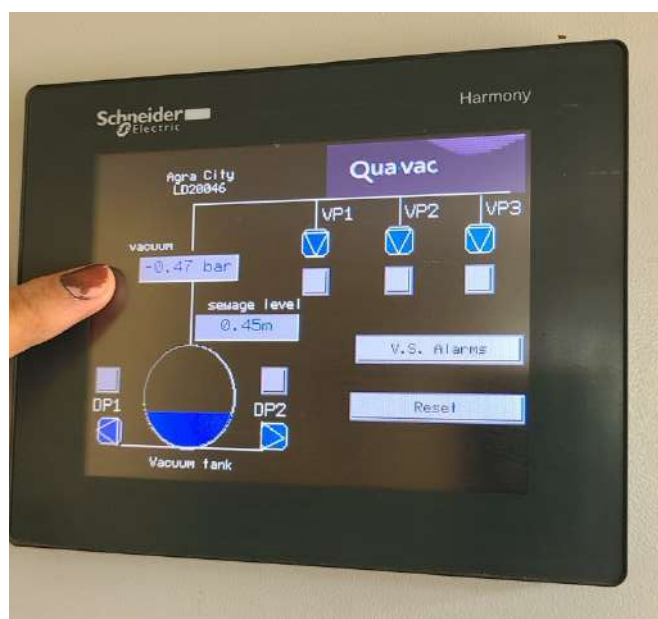
Fig 6: Display to monitor running of vacuum pumps and discharge pumps
