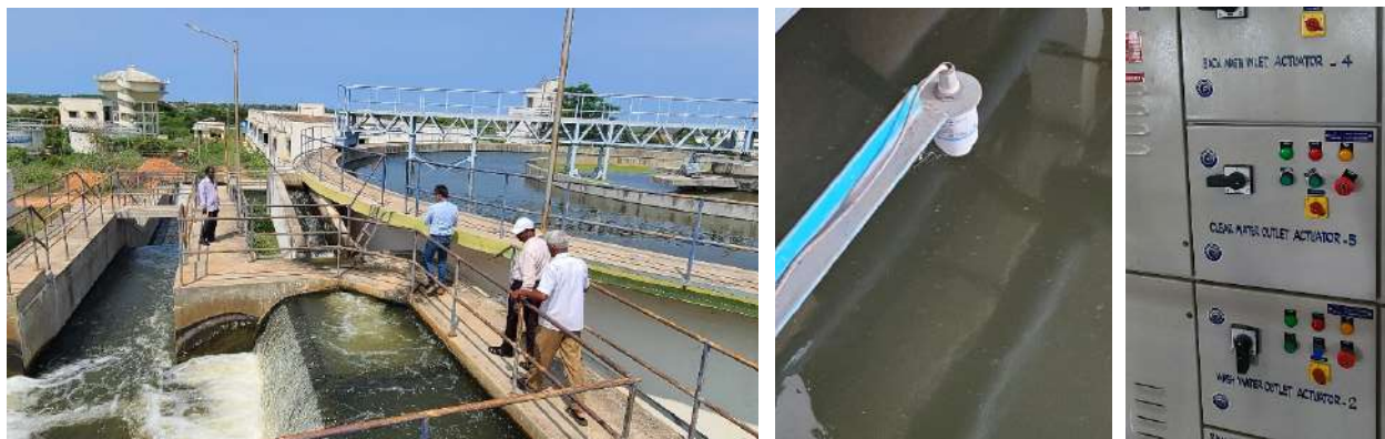
Figure 27: Visit to WTP by NIUA team (left), Level Sensor (Middle), Actuator Panel (Right)
