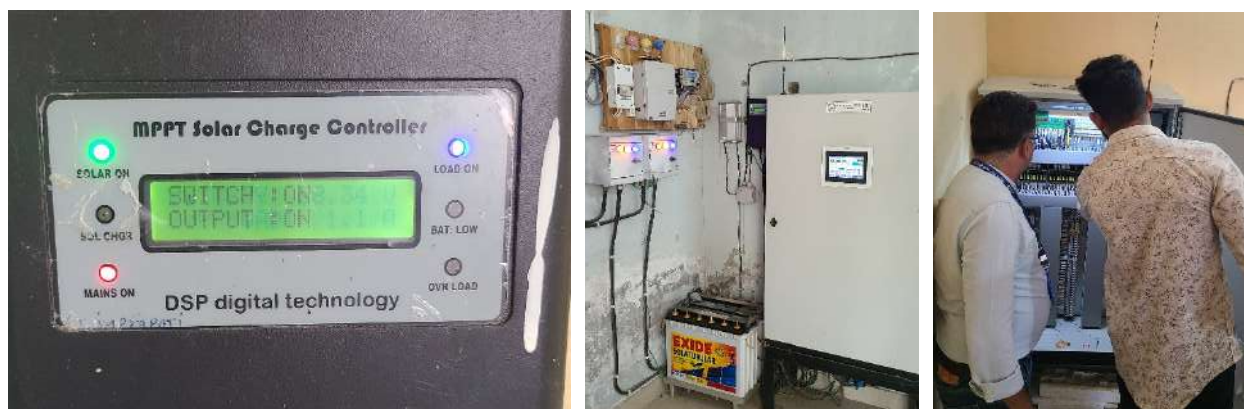
Figure 30: Solar battery panel (left), PLC panel with HMI (Closed pic-middle, open pic-Right)
