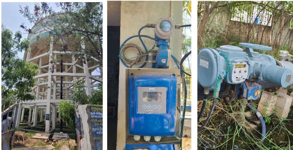
Figure 29: ELSR (left), Flowmeter and pressure transmitter (middle), Actuator (Right)
